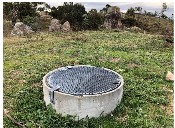
Water reticulation structure
